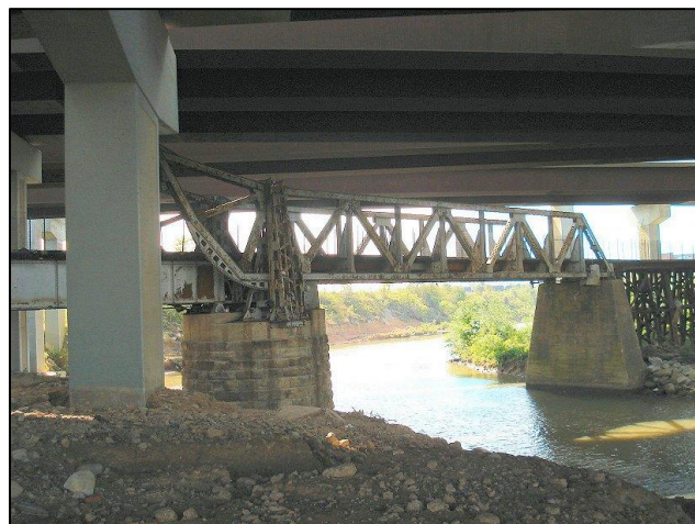
Figure 5: The Strauss Bascule Bridge is permanently fixed in its original location under the I-69 bridge over Buffalo Bayou. (Photo: Louis F. Aulbach)
